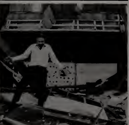
STONE AMONG THE RUBBLE — Chris Stone, president of Record Plant Los Angeles, stands among demolition of former Annex Studios in Los Angeles to be totally rebuilt to house the Record Plant companies. Move will be completed in the fall of this year.
