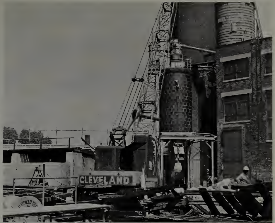
Rock-Ola plant modernization program in progress. An old rail trestle is no longer needed.
