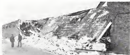
Here is a photo of the 200 ft. west wall which collapsed completely resulting in heavy exterior and interior damage, as well as personal injuries.
