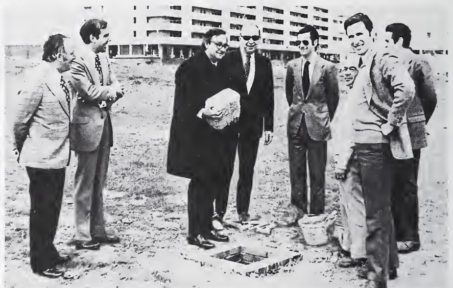
NEW RECORD PLANT —Discos CBS, CBS International's Spanish subsidiary, has begun construction of a factory near Madrid. CBS started operations in Spain in 1970. Shown here laying the cornerstone for the foundation of the new factory are Messrs. Kremer, Munoz (Managing Director of Discos Spain), De Rougemont (Vice President, CBS International European Operations), Wyngaard (Director of Operations in Austria, Switzerland and Spain) and engineers from the company constructing the building (shown L to R).
