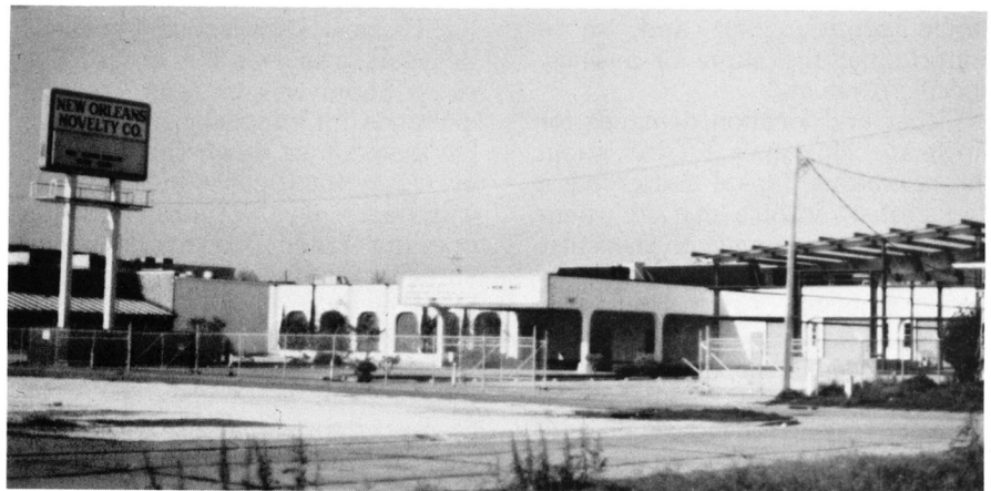
New Orleans Novelty Company, established in 1932, will move this summer from its old headquarters at 1055 Dryades Street to a new million-dollar complex at 3030 N. Arnoult Road in Metairie, Louisiana, in an area better known as Fat City. Shown under construction are the new loading docks of the distributing complex.
